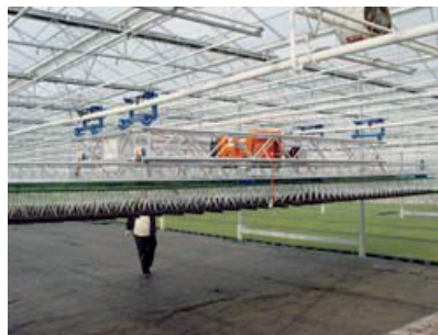
OVERHEAD CRANE SYSTEM
